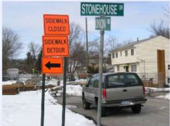
Stonehouse Drive Sewer Improvement project to begin as soon as updated plans are completed.
